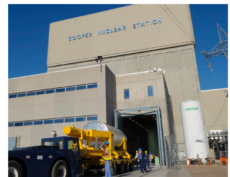
The cask exits the Reactor Building at CNS and begins down the heavy-haul road to the horizontal storage modules.
